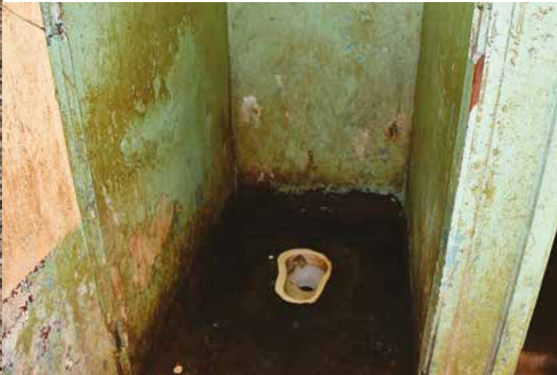
Toilet for patients and health workers in Kakamega
